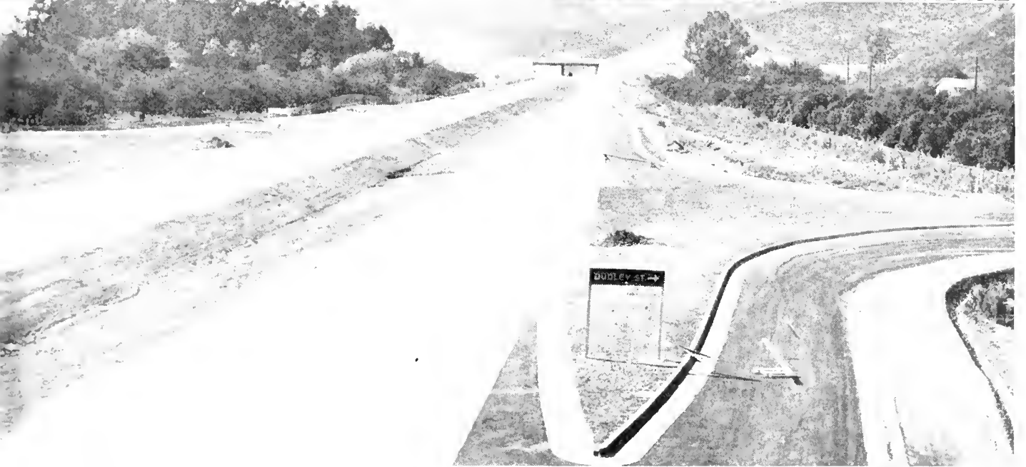
UPPER: Looking easterly along Ramona Freeway showing finishing-up operations in progress. CENTER: View along completed Ramona Freeway looking westerly from Ganesha Avenue Bridge showing Route 77/26 grade separation bridge and Kellogg Hills in background. LOWER: Looking westerly from Dudley Street Bridge showing completed Ramona Freeway with Ganesha Avenue Overcrossing in background.
